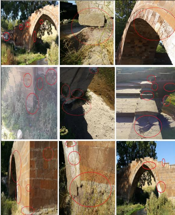
Figure 2. The observed damages in Emir Bayındır Bridge
