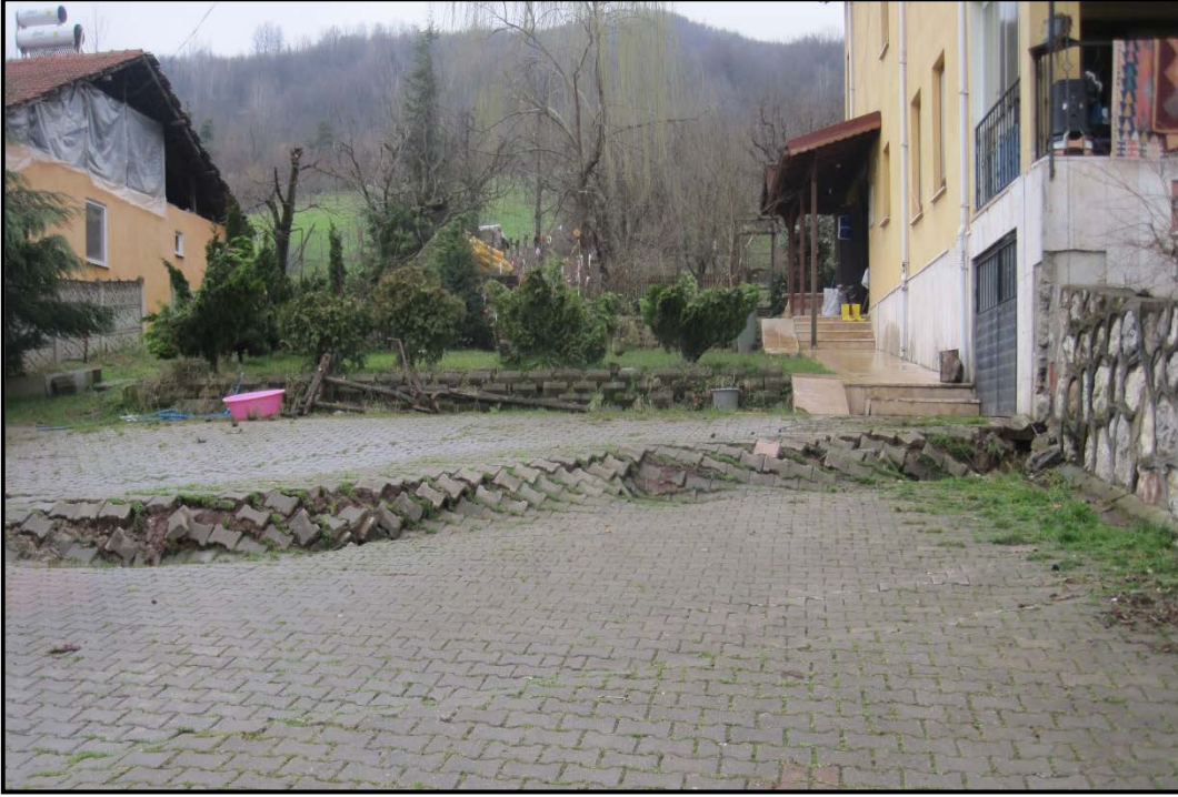
Şekil 8. Mamuriye köyünde zarar gören yol ve bina Figure 8. Road and building damaged by the landslide in Mamuriye village
