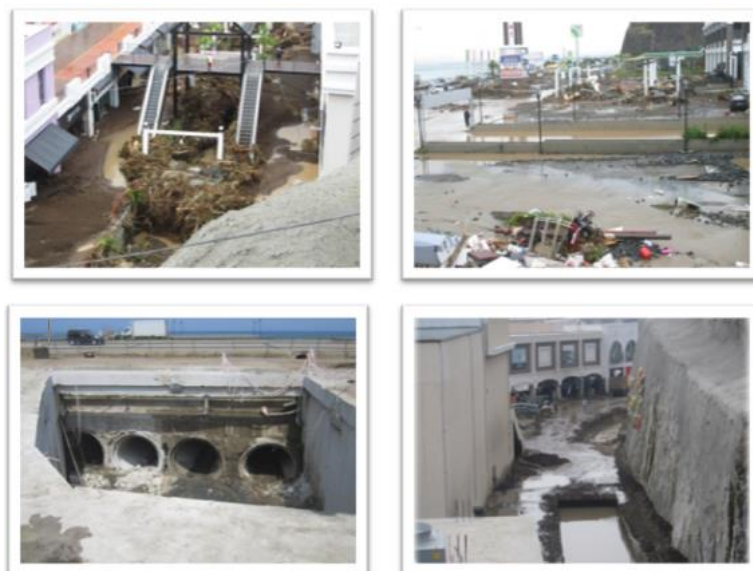
Figure 11. The Damage Caused by Incirli Stream Flood to the Shopping Mall
