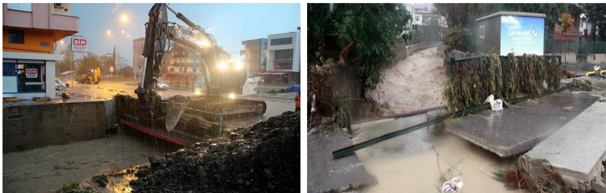
Figure 15. Flood Damage (Highway Bridge) and in Atakum Coastal Road Bridge
