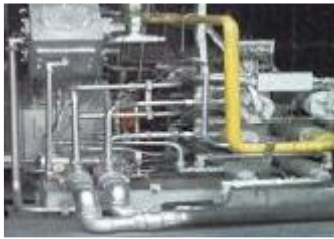
Figure 1. Gas Compressors with High Pressures
