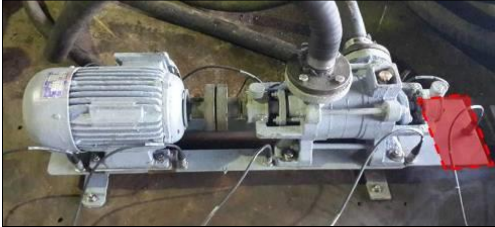
Figure 2. Electric Motor Driven Pump Set-up
