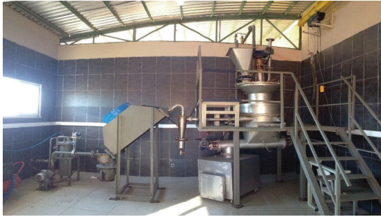
Figure 2- General view of gasifier system
