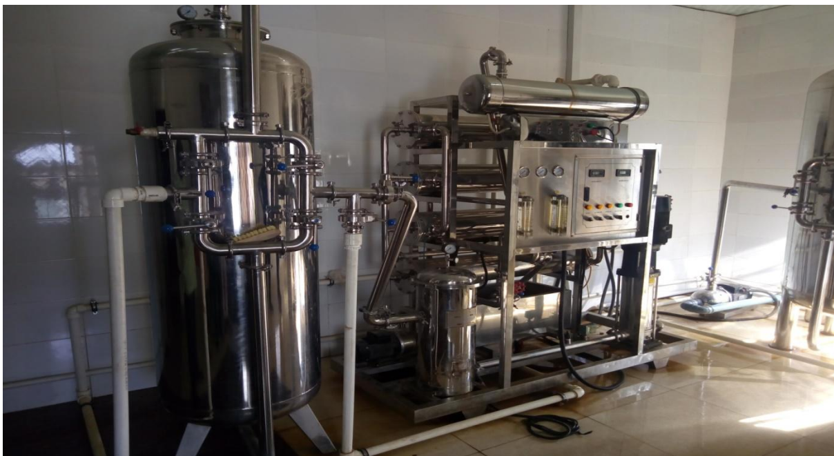
Plate 1: Reverse Osmosis Unit of one of the Sampling Points
