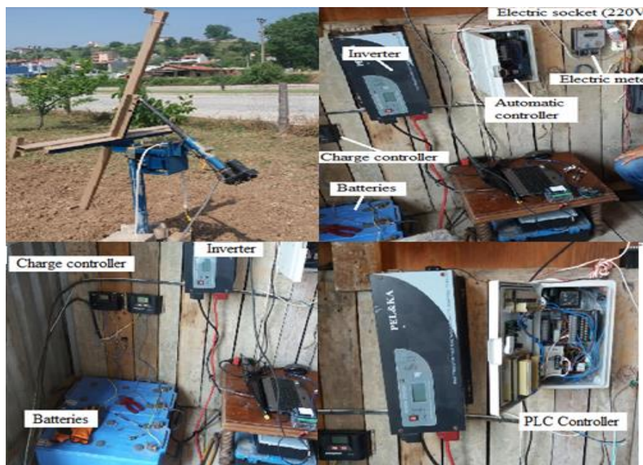
Figure 6. All apparatus (inverter, batteries, electric meter, data logger and etc.) used in the experiment
