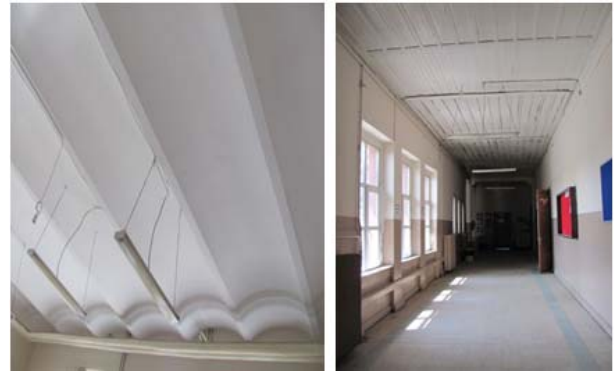
Figure 7 - Ceiling in ground floor classrooms and corridor to which classrooms are opened
