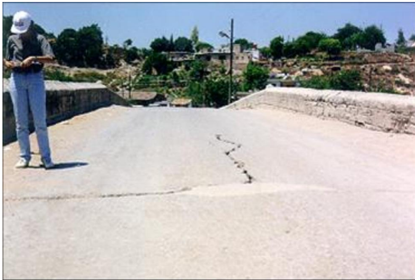
Figure 3: Damages occurred in superstructure of the Misis Bridge during the 1998 Adana-Ceyhan earthquake (Ural et al. 2008)
