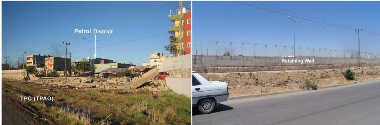
Figure 14. Retaining wall of Turkish Petroleum Corporation facilities demolished in the flood event on October 31-November 1 2006 and later rebuilt.
