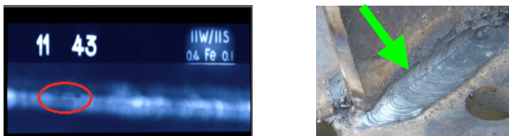
Figure 2. longitudinal crack and Radiography film image that longitudinal crack specified in it
