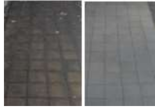
Figure 15. Decreased Ability to Absorb Moisture due to the Use of Nano-Based Water Resistance Coatings, and Followed by Reduce the Risk of Levee Moss and Algae Growth
