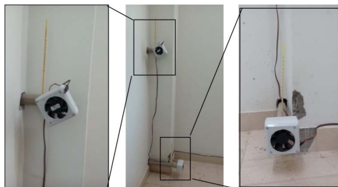
Fig.4. Heating system in room, on left warm air entering into room from collector while on right cold air exhausts from room entering into collector.
