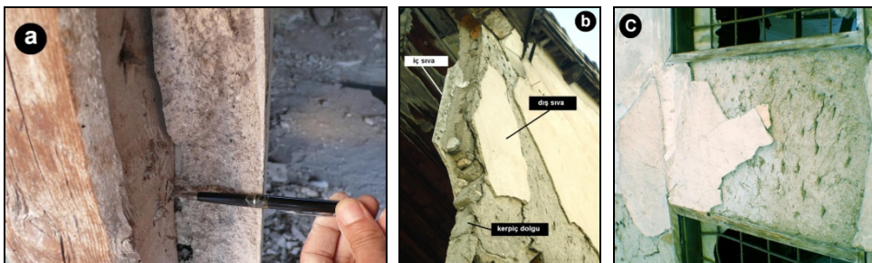
Figure 2. [a,b] Coarse and thin plaster layers, [c] chamfered surfaces on which plasters are applied.
