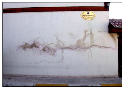
Figure 4. Crackles, spillages and salt effects observed at cement binding plaster used on the restored façade of Abdi Ağa Residence.
