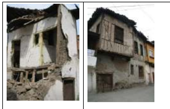
Fig.9. The examples for deterioration
