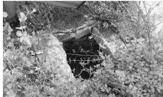
Figure 4. A view from the well in the courtyard of Atik Valide Sultan Hospital [16]
