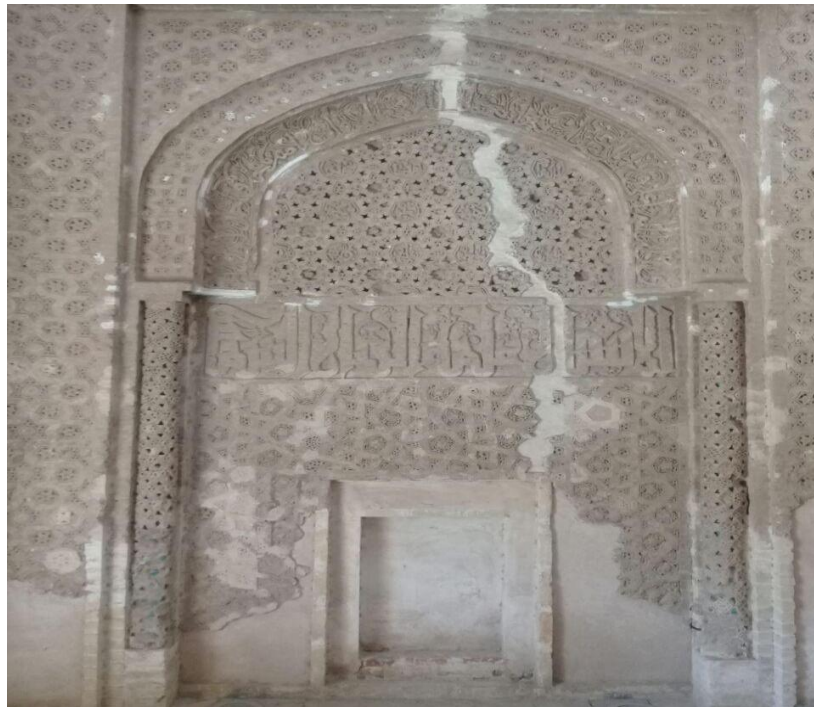
Figure 13: A view of the west side of Khaje Atabak's Tomb after the primary restoration (photo taken by the writer)
