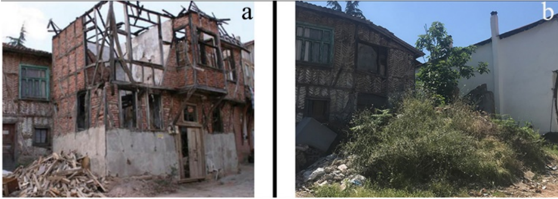
Figure 7: The heavily damaged building (a) was completely lost in 2018 (b).
