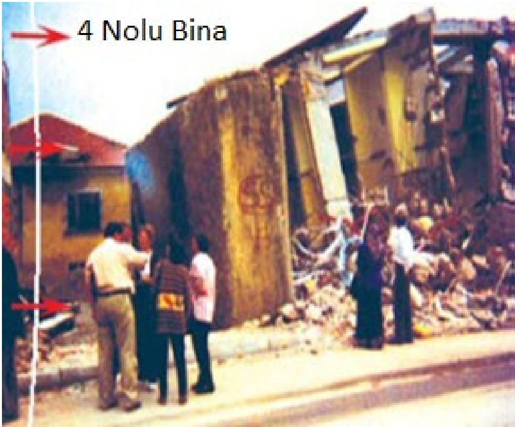
Şekil 9. Devrilen 4 Nolu Bina (Yükseklik:12.00 m, Genişlik:6.00 m) [1] (Overturned Building #4 (Height:12.00 m, Width:6.00 m))
