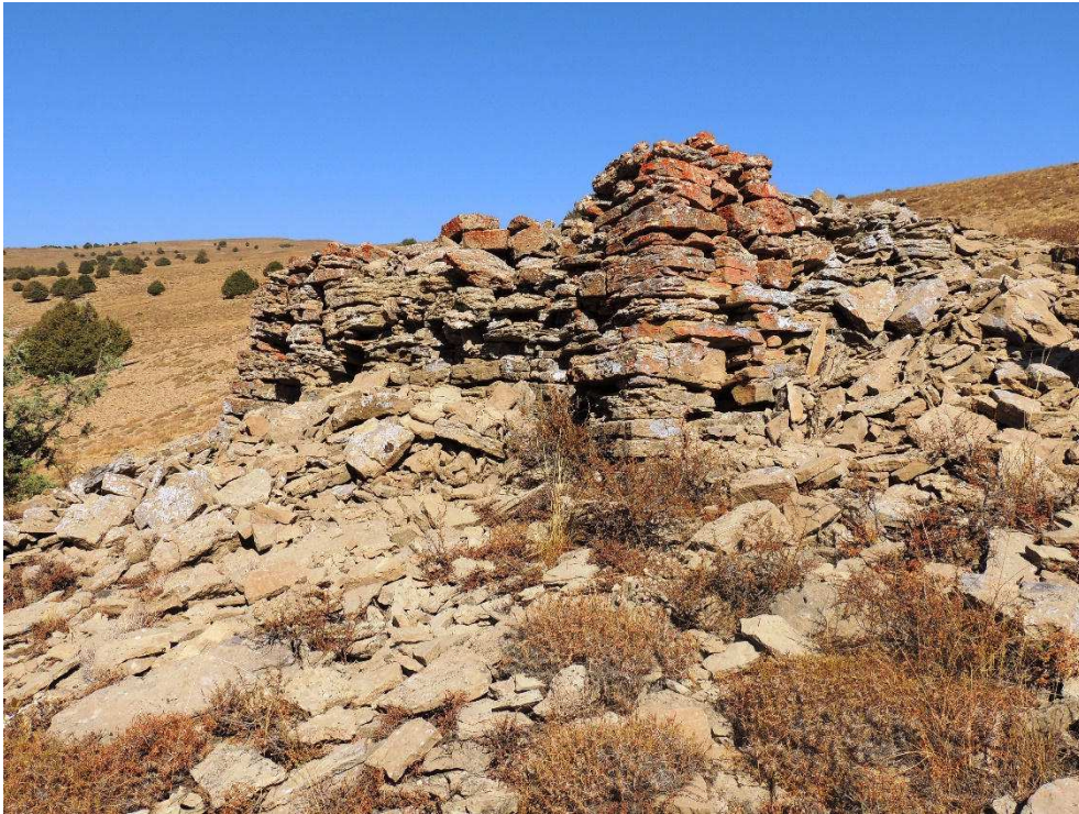
Fig. 39 Destroyed facade of a construction.
