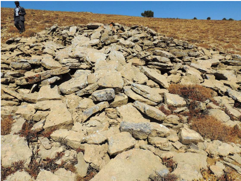
Fig. 40 One of the destroyed construction.
