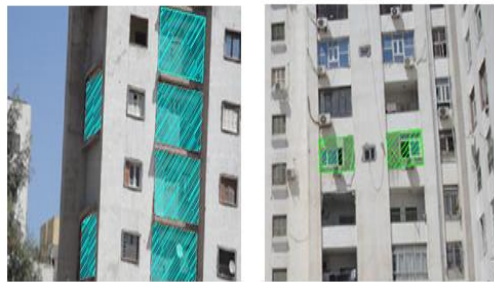
Closed the balconies by users- Air-Port Road Housing project
