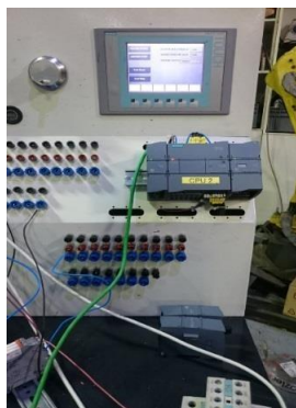
Figure 5. Siemens SIMATIC S7-1200
