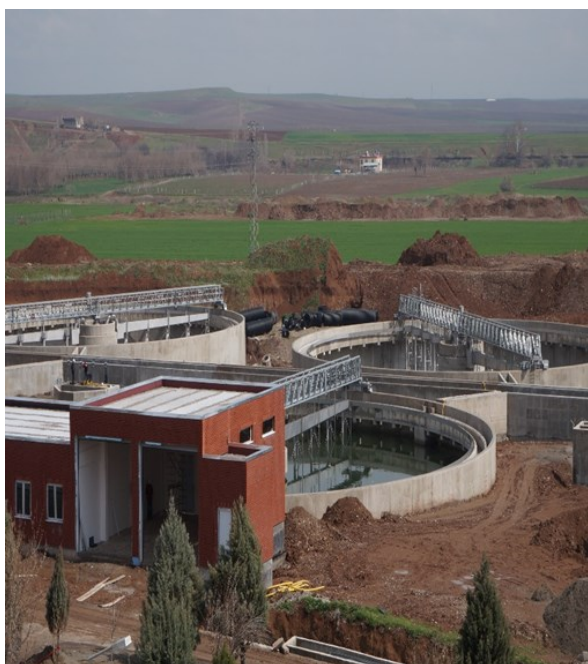
Figure 5: Diyarbakır biological water treatment open-air facilities
