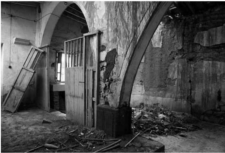
Fig. 12 Khan, Building G (coffee house), view from southern bay towards northern wall, souventza (cornice) on wall to left, middle pillar reinforced by concrete cover
