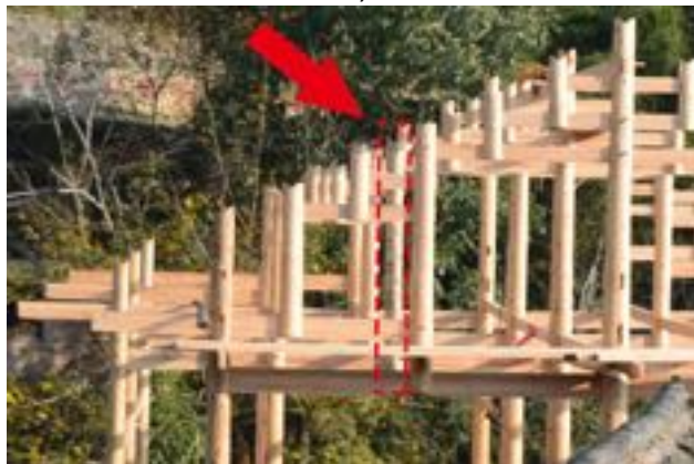
Figure 5. Short column marked with numerous ink lines, Dali Villiage, 18/11/2016
