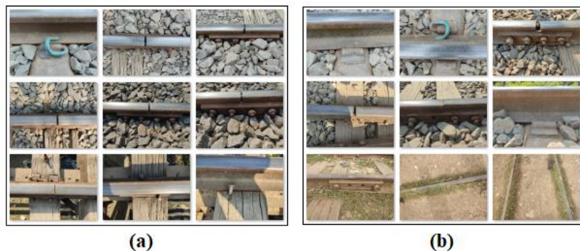
Figure 1. Dataset classes and sample images; a) Non-defective images, b) Defective images
