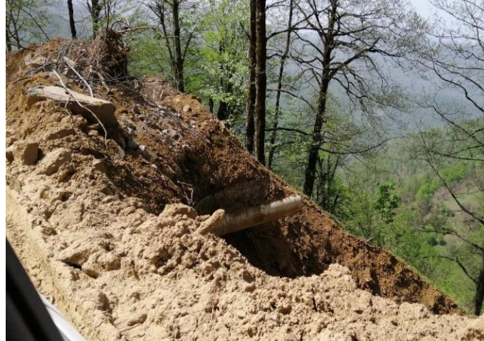
Figure 8. Severe erosion of the output of the old waterway
