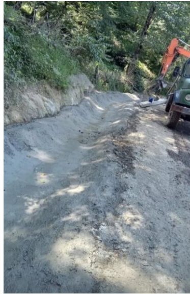
Figure 15. The concrete lining of the ditches without meeting the required minimums (2023 Summer)
