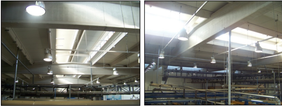
Figure 3a and 3b. Sunlight gaps that are left on the roof production area.
