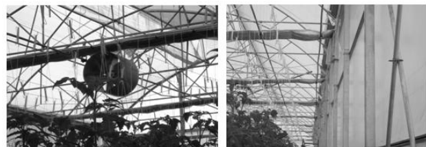
Figure 3. The modern greenhouses farm used circulation fan and thermal screen.
