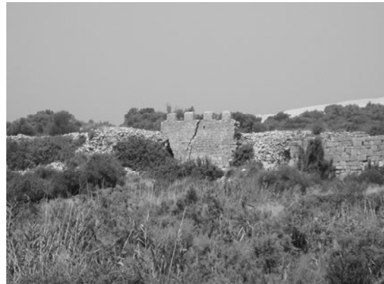
Fig. 7. The outer face of the medieval city wall restored by the Seljuks
