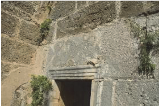
Fig. 14: The indications and in situ remains of the two roofs remaining on the lintel.
