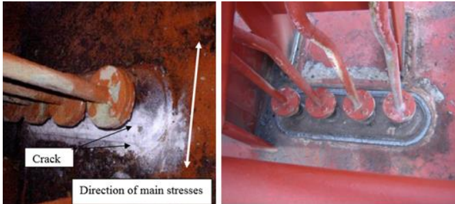
Figure 4. Crack in way of pipe penetration in main deck [2].
