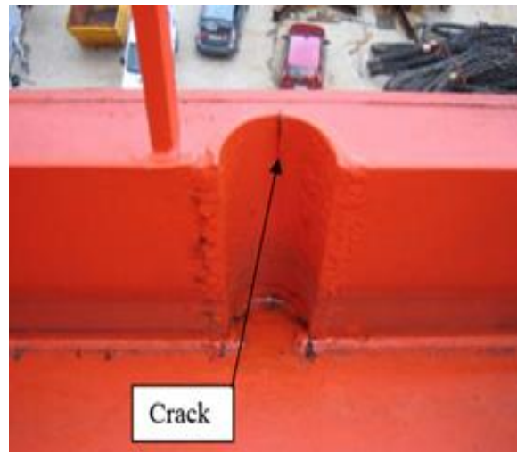
Figure 12. Cracks in gutter bar (in closed view).
