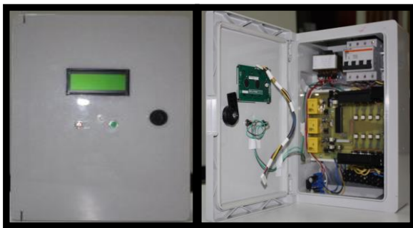
Figure 11. The boxed designed starter and protection relay and its layout of the elements.
