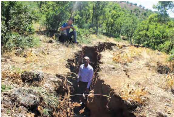
Figure 8- Large cracks were formed at Çaytepe Duşmalan Locality, the east of Genç, due to the slide that occurred in early summer of 2017.
