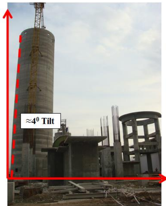
Figure 7. Tilting of clinker silo
