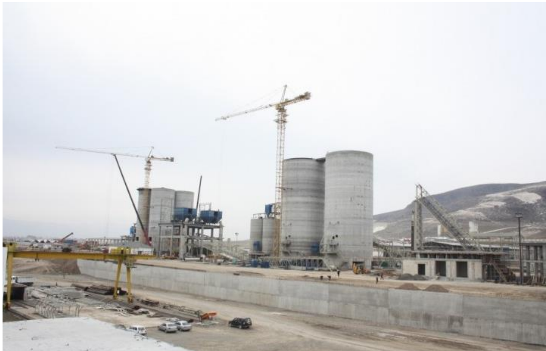
(b) A view during construction from west side of the plant Figure 2. West side of the construction area ( \approx 850\text{m} \times 900\text{m} )
