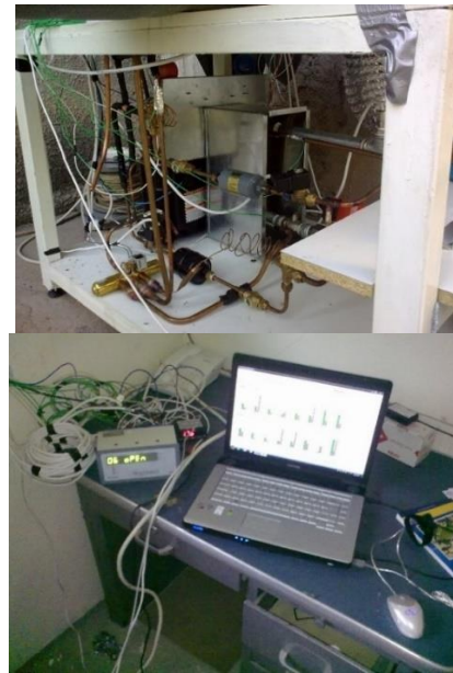
Figure 2. General view of the experimental setup used for space heating applications in GSHP
