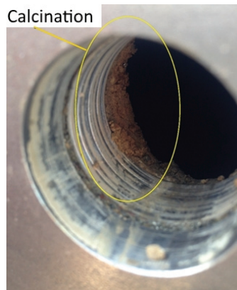
Figure 2 - Calcination in the pipe seen from a sensor tap
