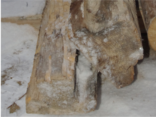
Fig. 8 - Timber joists with an inverted T-cross section from a demolished timber floor
