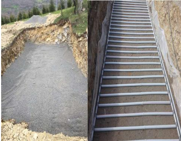
Figure 1. Artificial pond and underground pipe setup [10]
