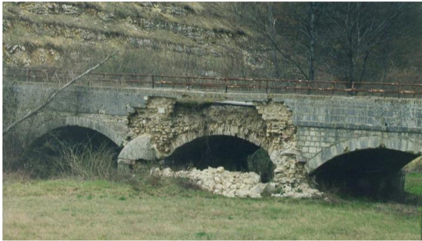
Figure 2: Collapse of spandrel of a masonry bridge during the 1997 Umbria-Marche earthquake
