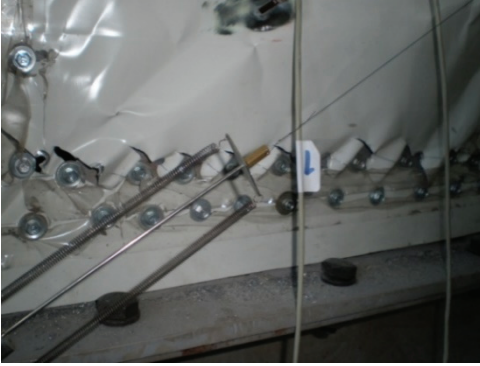
Figure 26 - 7\delta_y ; front side plate-to-frame connections on the left, torn from the screw edges
