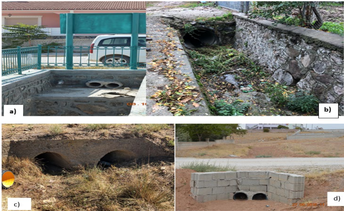
Figure 7. Narrowing the flood protection structures of a) Kirkpinar region, b) Gevrekli region, c) Yesilyurt region), Yeniceoba region
