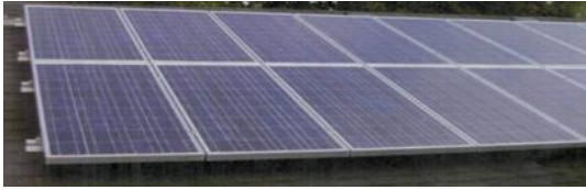
Fig 1. A typical PV Array Individual modules are attached to a racked system and wired together to form an array [10].
