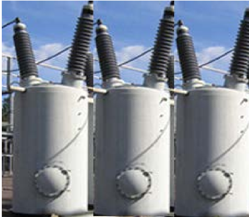
Figure 1. Circuit breakers in transformer centers.
