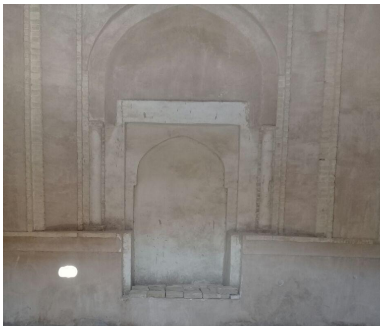
Figure 19: A view of the north side of Khaje Atabak's Tomb which had undergone great damage (photo taken by the writer)
