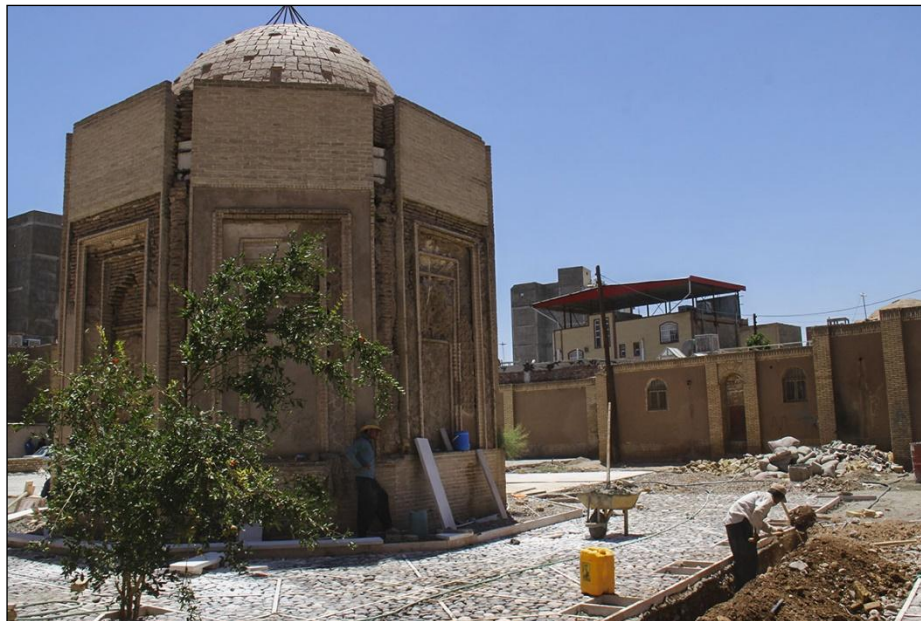
Figure 7 and 8: Construction of the cobbled yard (photo taken by the writer in 2016)
