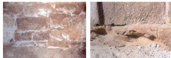
Figure 5. Damage caused by salting and freezing-thawing of stones
