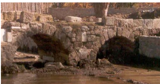
Figure 4. Damage to the historical Dortgoz Bridge on the road route
