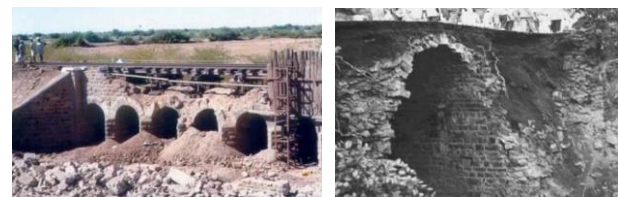
Figure 2. Bridges damaged by the 2001 Bhurj earthquake and the Koyna earthquake in India
