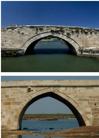
Figure 7. Deformed arch after repair, Buyukcekmece Bridge
