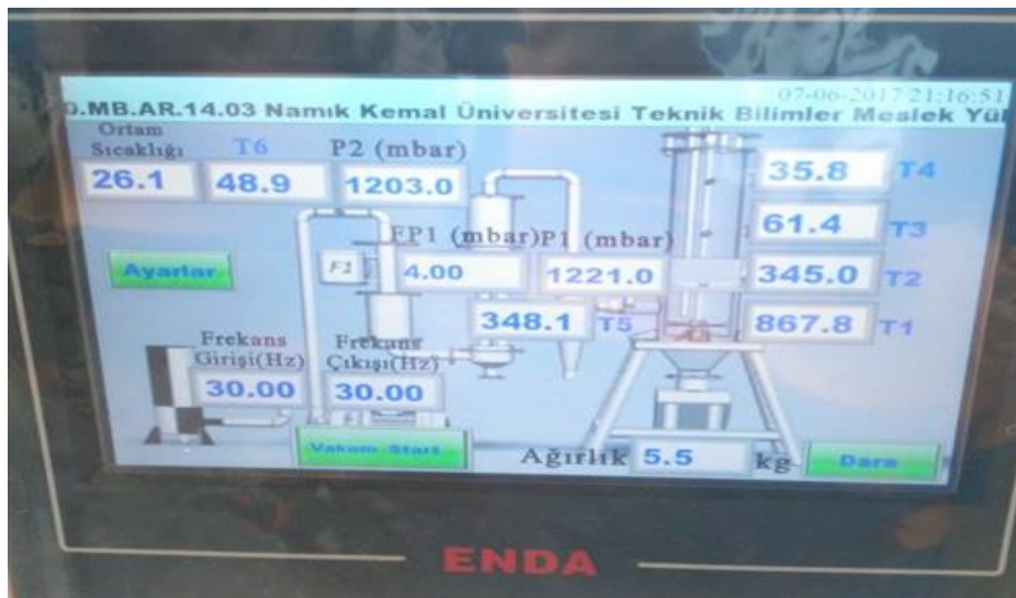
Figure 6. Measurement and control equipment display screen
