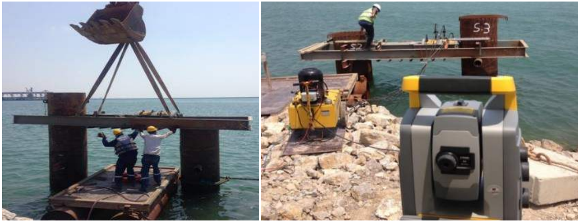
a. Implementation of the Reference Beam b. Topographical Survey Equipment Figure 5. Setup of the Field Test
