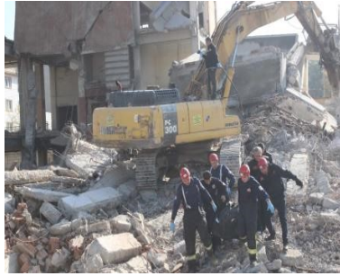
(a) Demolition accident in Denizli
