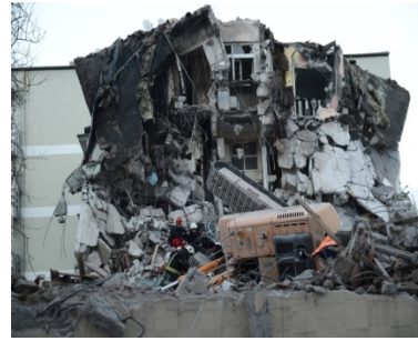
b) Demolition accident in Malatya
