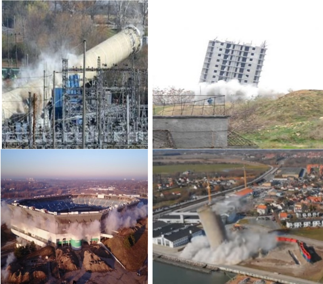
Figure 5. (a) Toppling of the Power Plant in the wrong direction, (b) Demolition of the structure in the not intended direction, (c) Demolition of the structure in the not intended direction, (d) Toppling of the silo in the wrong direction.
