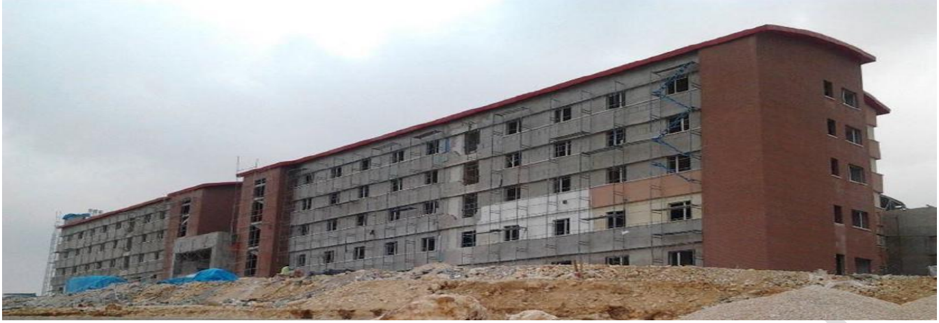
Picture 1. Kayseri Reception and Accommodation Center
